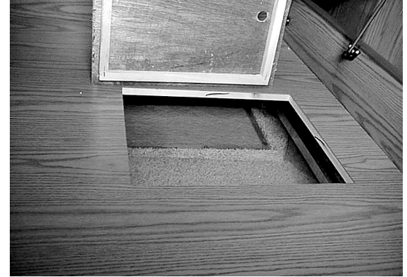
AC Filter under mattress board
