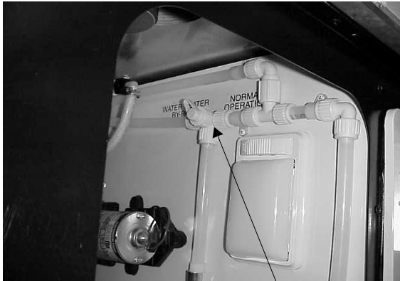
Water Heater Bypass Valve
