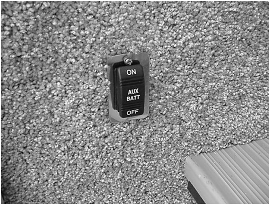
Aux. Batt. Disconnect Switch in Entrance Stepwell
