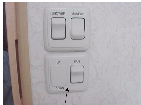
Bath Vent Controls
