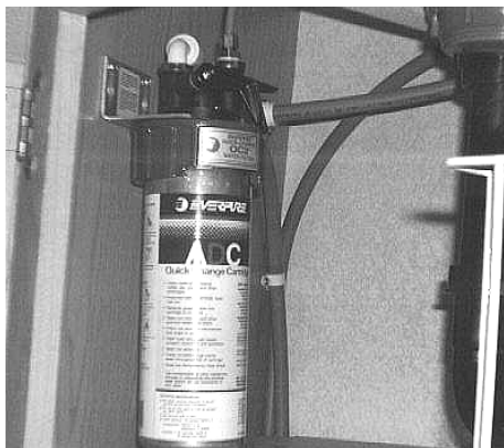
Water Filter Assembly - Below Galley Sink
