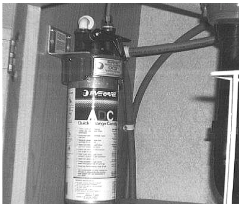
Water Filter Assembly - Below Galley Sink
