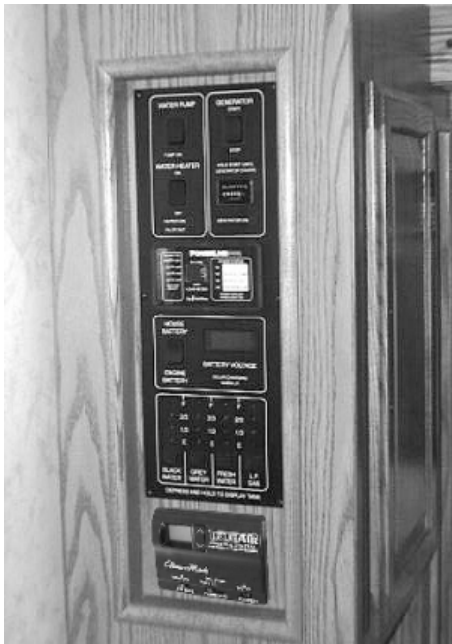
One Place Monitor Panel
