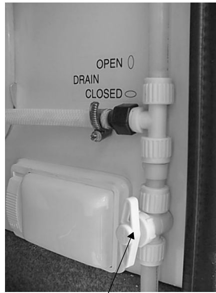
Water Line Drain Valve
