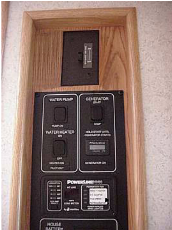
Powerline™ EMS Status Panel
