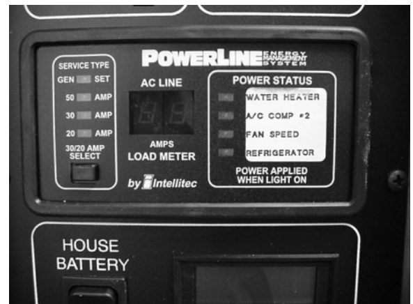
EMS Display on Monitor Panel
