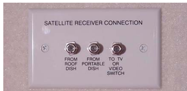
Satellite TV Receiver Connection (in front video center cabinet)
