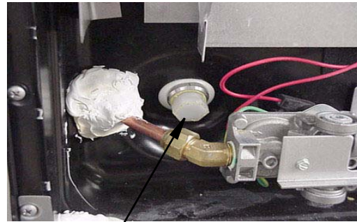
Water Heater Drain Plug Remove with socket
