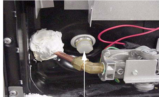
Water Heater Drain Plug (Remove with socket)
