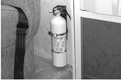
Fire Extinguisher (typical installation - your coach may vary according to model and floorplan)
