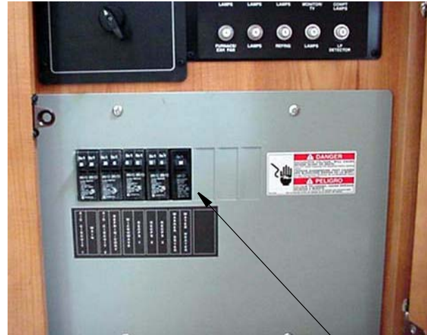
120-Volt House Circuit Breakers
