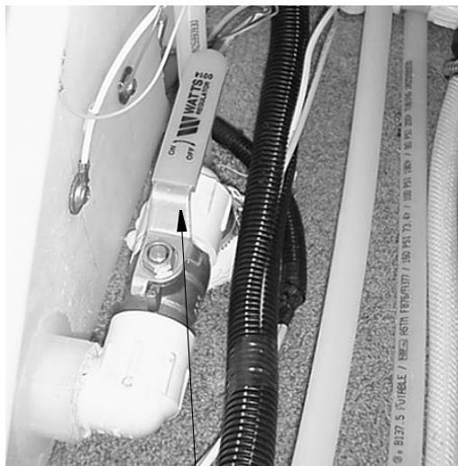
Water Tank Drain Valve (Typical)
