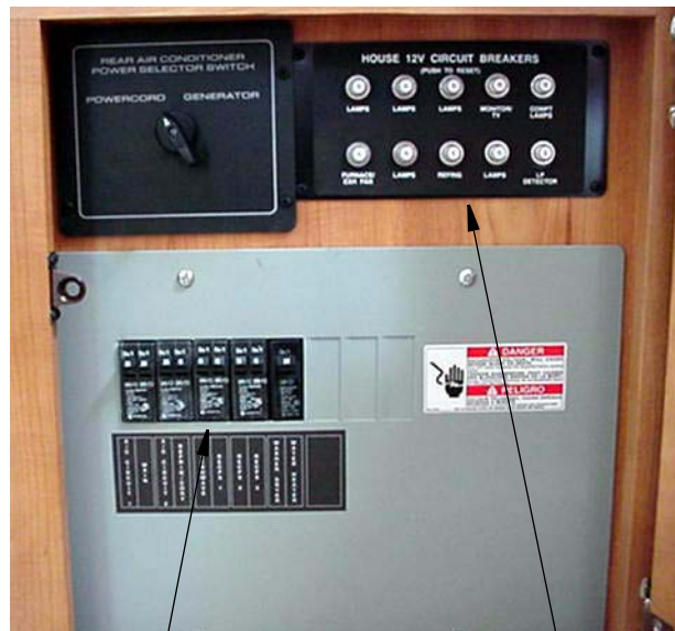
120-Volt House Circuit Breakers 12-Volt House Circuit Breakers
