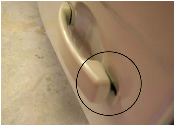
Door Unlatched (note gap)
