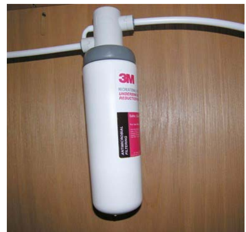
Cold Water Filter Assembly below Galley Sink (Hot water line is not filtered.)
