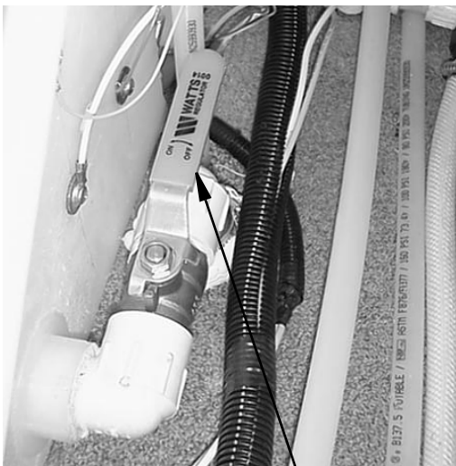
Water Tank Drain Valve (Typical)
