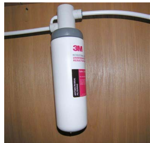
Cold Water Filter Assembly below Galley Sink (Hot waterline is not filtered)
