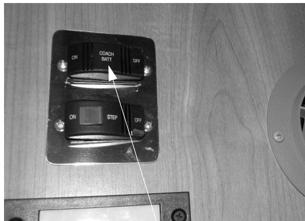
Aux. Batt. Switch - Typical (Located near entrance door)
