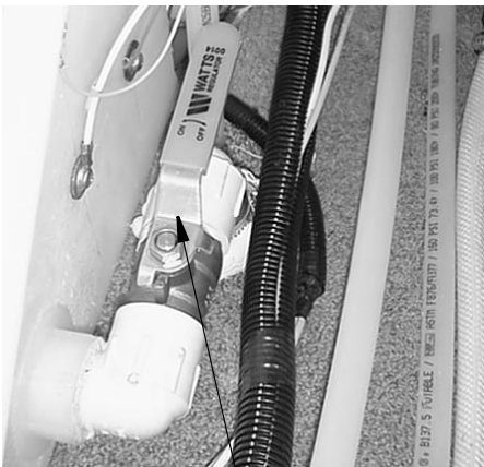
Water Tank Drain Valve (Typical)
