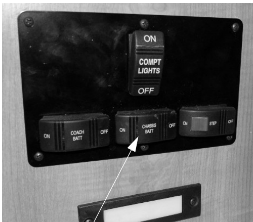
Chassis Battery Disconnect Switch (located inside the entrance door)
