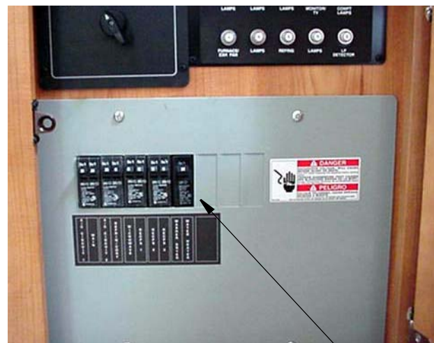
120-Volt House Circuit Breakers
