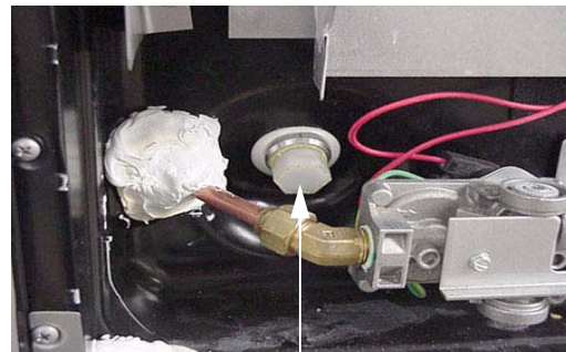
Water Heater Drain Plug (Remove with socket)
