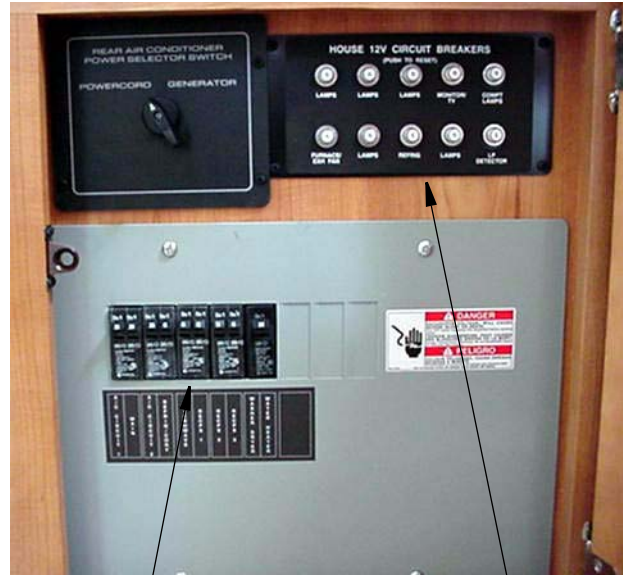
120-Volt House Circuit Breakers
