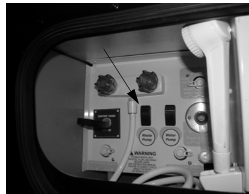
Waste Pump Switch (Located in water service center) -Typical View
