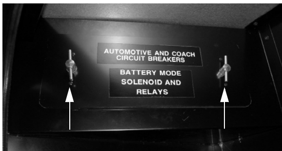
Chassis and House 12V Breaker Panel (Located in passenger side compartment) -Turn both latches to remove cover
