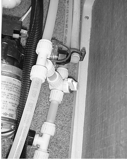
Waterline Drain Valve (Located behind access panel in rear storage compartment) -Typical View
