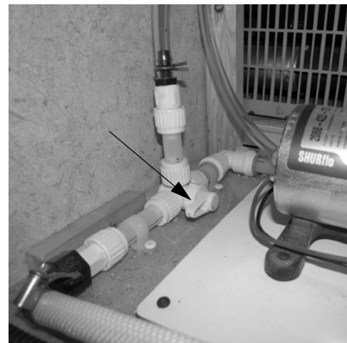
Winterization Valve -Typical View
