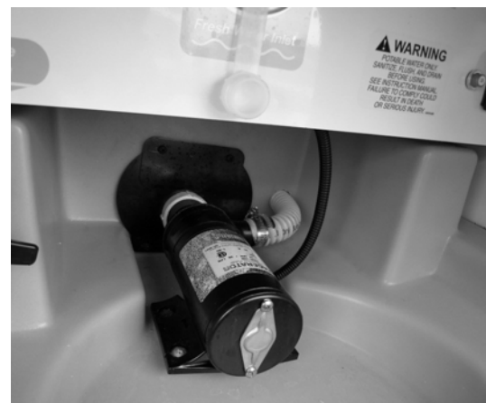
Waste Pump (Located in water service center) -Typical View
