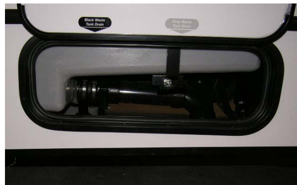
Holding Tank Dump Valves (Located in mid-driver side access compartment) -Typical View
