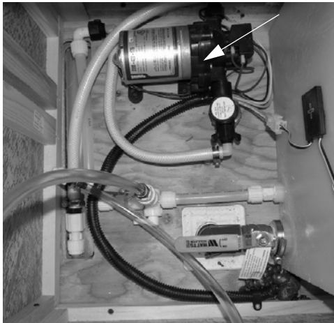
Water Pump (Located beneath bed - lift mattress to expose access hole) -Typical View
