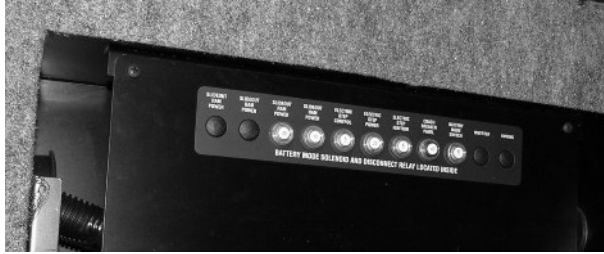
Chassis and House 12V Breakers (Located in passenger side compartment) -Typical View * Shown with cover removed
