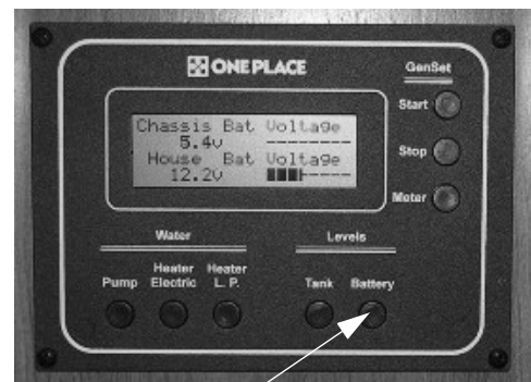
Battery Levels Switch
