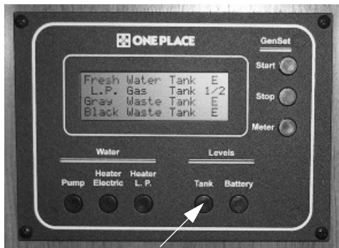
Tank Levels Switch
