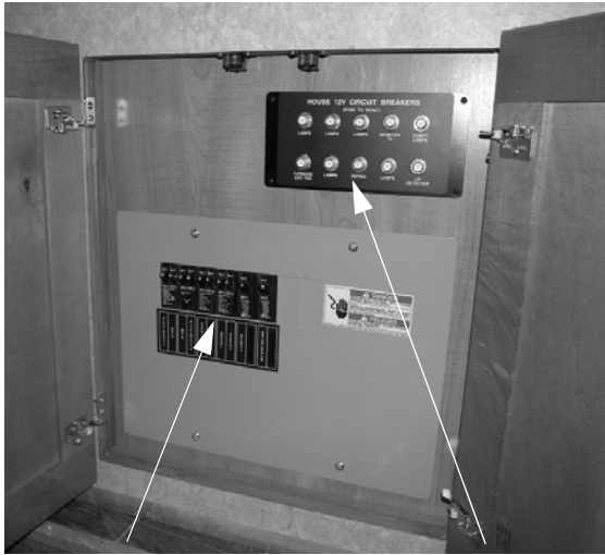
120-Volt House Circuit Breakers
