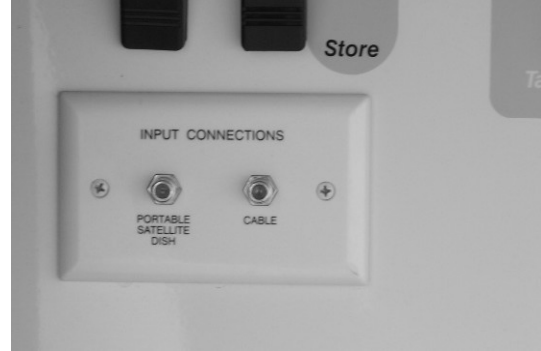
Exterior Connections for Satellite Dish and Cable TV (Located in water service center) -Typical View
