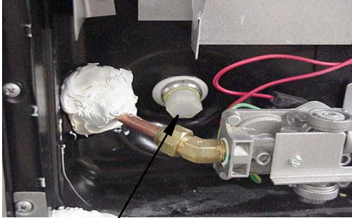
Water Heater Drain Plug (Remove with socket)
