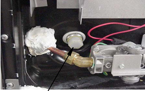
Water Heater Drain Plug (Remove with socket)
