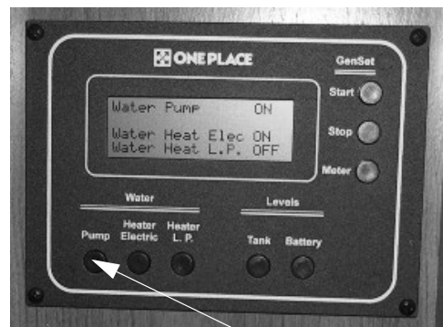
Water Pump Switch
