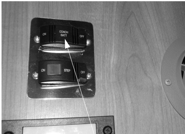
House/Coach Battery Disconnect Switch
