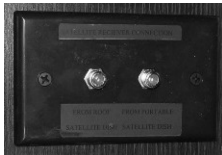
Interior Connection for Satellite Dishes (Located in cabinet or on a wall near TV) -Typical View
