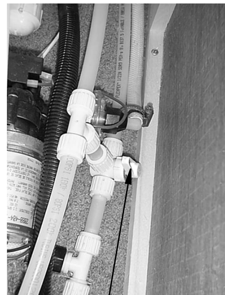
Waterline Drain Valve (Typical)
