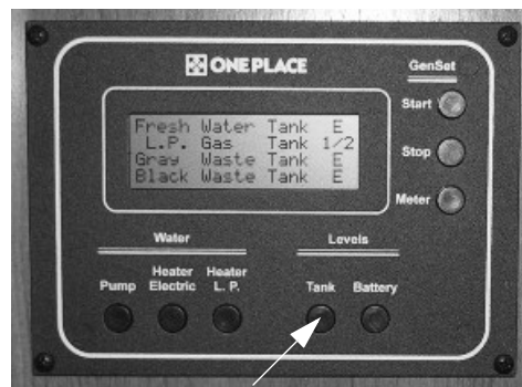
Tank Levels Switch
