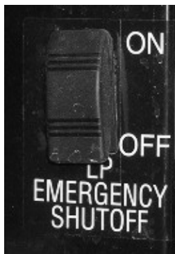
Main Tank Shutoff Switch (Located in driver side compartment) -Typical View
