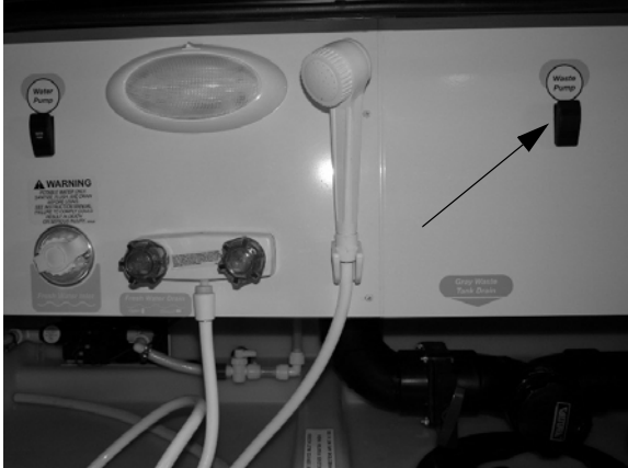
Waste Pump Switch (Located in water service center) -Typical View
