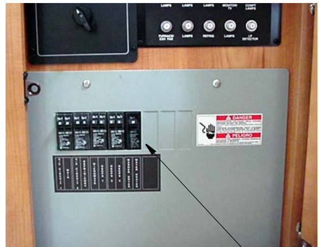
120-Volt House Circuit Breakers -Typical View
