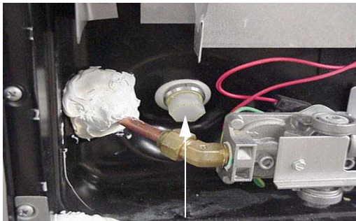
Water Heater Drain Plug (Remove with socket)
