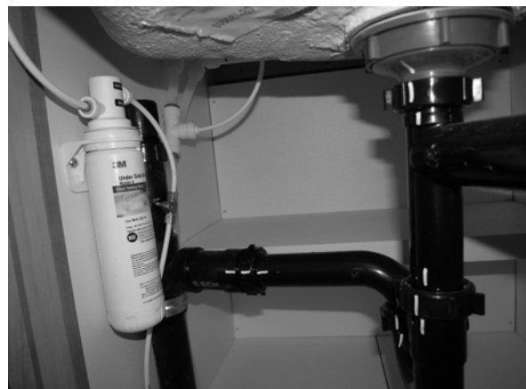
Ice Maker Filter Assembly (Located below galley sink)
