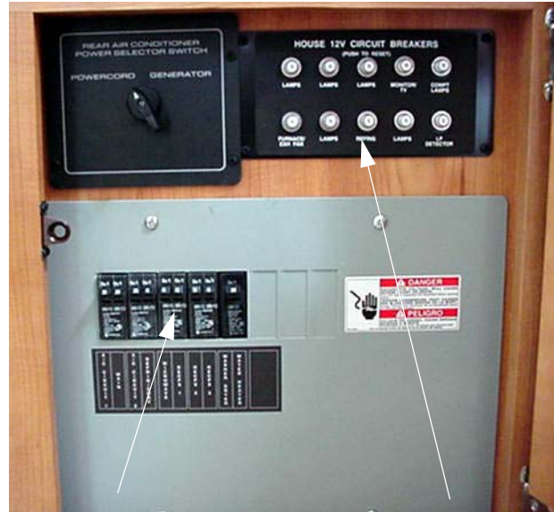
120-Volt House Circuit Breakers 12-Volt House Circuit Breakers
