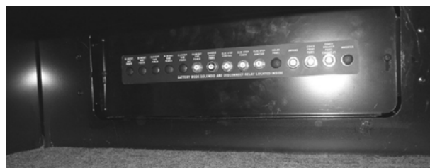
Automotive Chassis and House 12-Volt Circuit Breakers (Located inside passenger compartment) -Typical View
