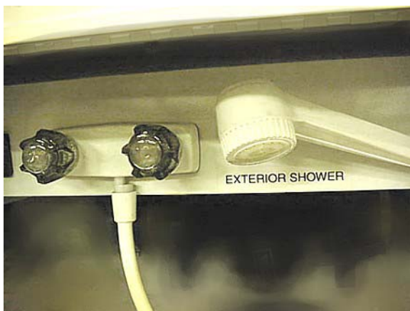
Exterior Shower/Wash Station -Typical View
