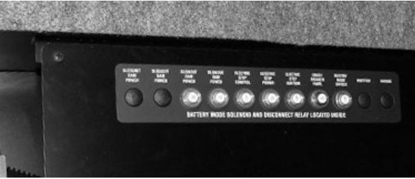
Automotive Chassis and House 12-Volt Circuit Breakers (Located inside passenger compartment) -Typical View
