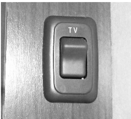
Bedroom TV 12-Volt Master Power Switch (Located on cabinet or wall near TV) -Typical installation shown
