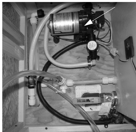
Water Pump (Located beneath bed - lift mattress to expose access hole) -Typical View
