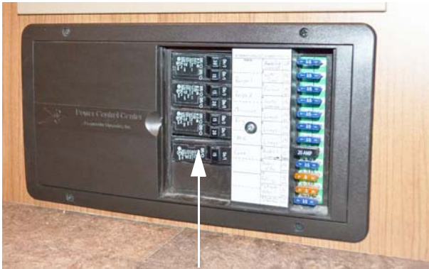
120-Volt Circuit Breakers -Typical View
