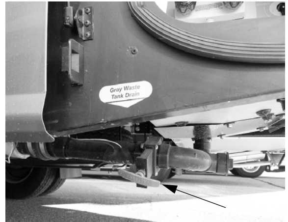
Gray Waste Tank Drain Valve (Located beneath rear driver side of coach) -Typical View
