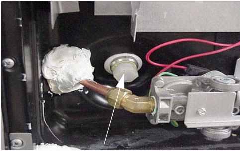
Water Heater Drain Plug (Remove with socket)
