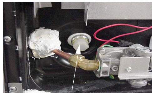
Water Heater Drain Plug (Remove with socket)
