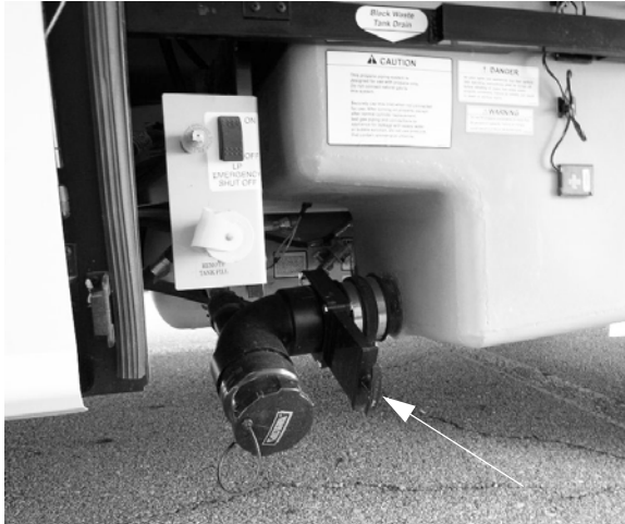
Black Waste Tank Drain Valve (Located in driver side compartment) -Typical View
