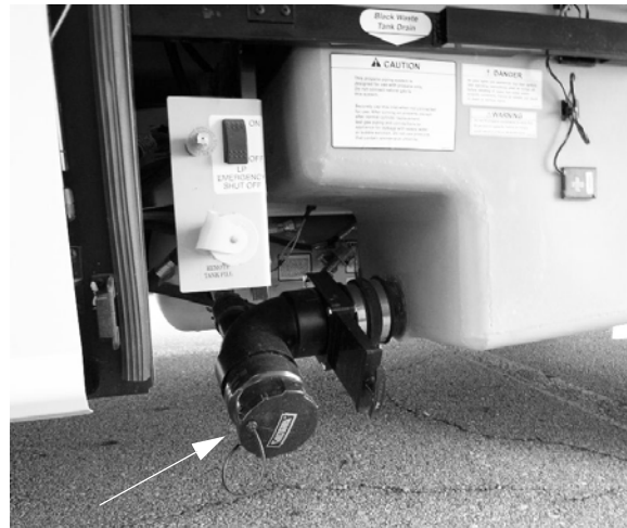
Sewage Drain Outlet/Dust Cap (Located in driver side compartment) -Typical View
