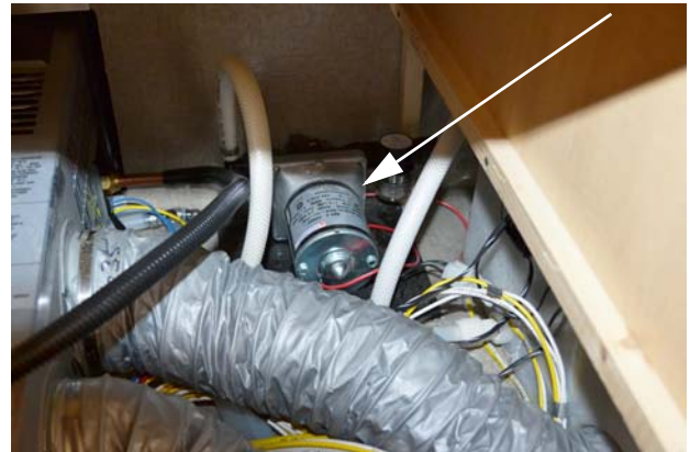
Water Pump • Model 23T - located beneath galley (remove panel to access) -Typical View
