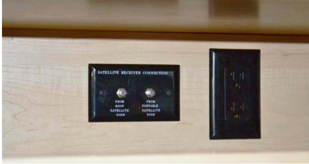
Interior Connection for Satellite Dish (Located in cabinet behind front overhead TV) -Typical View
