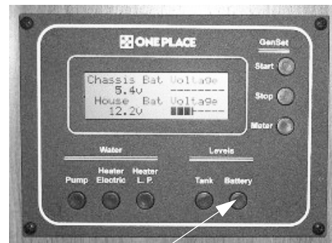
Battery Levels Switch
