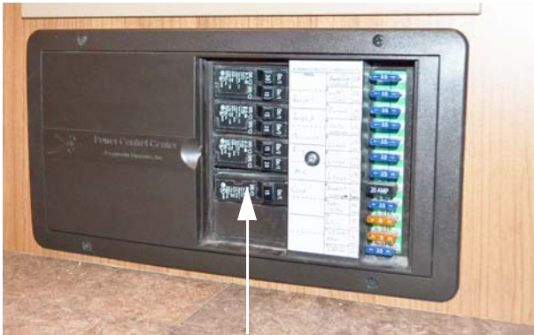
120-Volt Circuit Breakers -Typical View
