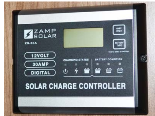
Solar Charge Controller (Located near monitor panel)
