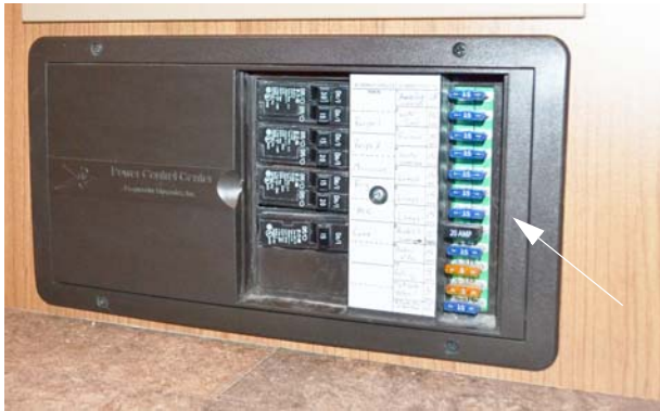
House 12-Volt Fuses (Located on right-hand side of Power Converter) -Typical View
