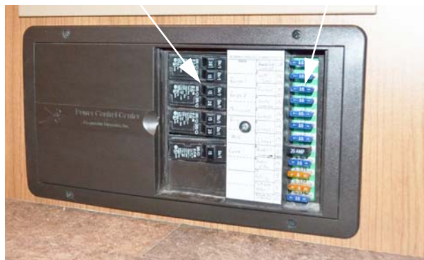
Power Center (Converter) -Typical View
