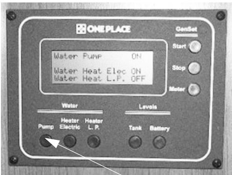
Water Pump Switch
