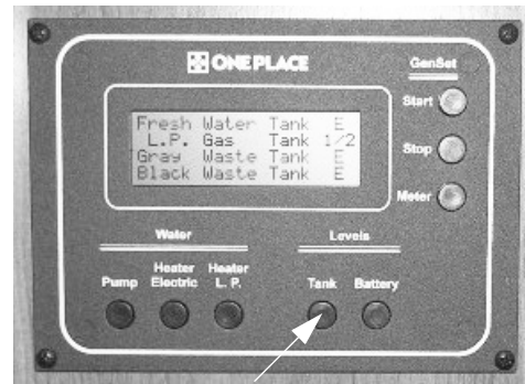
Tank Levels Switch
