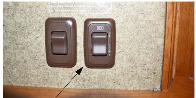
Power Lift/Lower Control Switch (Located near bedroom nightstand) -Typical View
