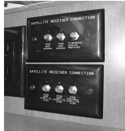
Interior Satellite Dish Connections (Located in the entertainment center cabinet) -Typical View
