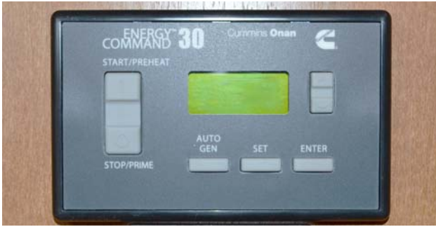
AGS Control Pad (Located near monitor panel)
