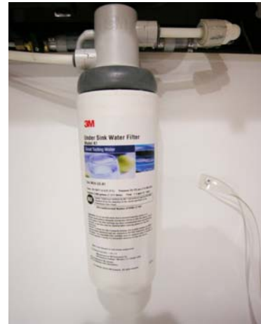
Galley Filtered Cold Water Faucet/ Ice Maker Filter Assembly (Located below galley sink) -Typical View
