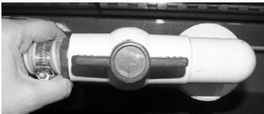
Sewage Drain Hose Valve
