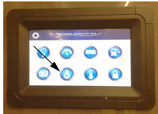
Water Pump Switch
