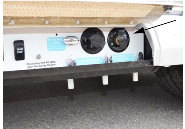
Black Waste Tank Flush Inlet (Located in water center compartment) -Typical View
