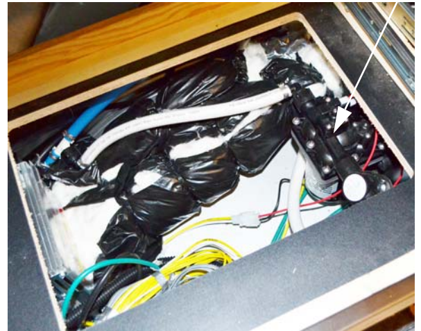
Water Pump (Located beneath bottom wardrobe drawer, remove drawer to access)
