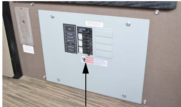
120-Volt Circuit Breakers -Typical View
