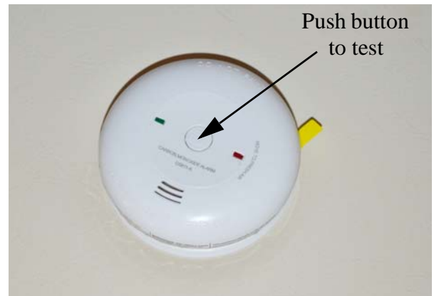
Carbon Monoxide Alarm
