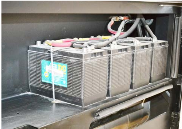
House/Coach Batteries -Typical View
