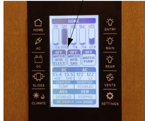
Water Heater Switch “HOME” Screen (Located on Multiplex Monitor Panel)
