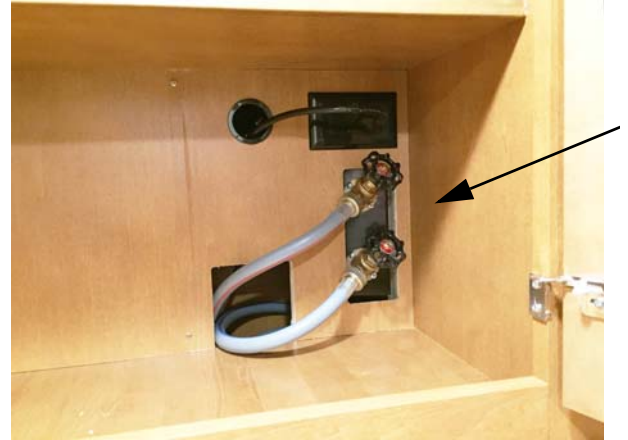
Water Supply Faucets (Located inside cabinet above washer) *Model 38W
