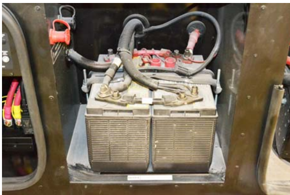
Chassis Batteries -Typical View
