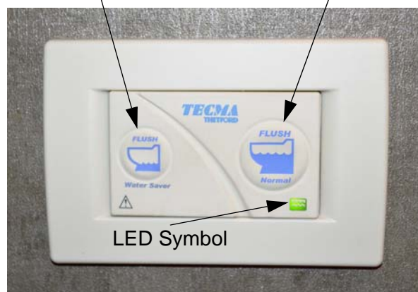
Wall Switch/Controller (Located on wall near toilet)
