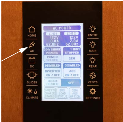
Generator Switch and Hourmeter (Located on multiplex monitor panel “AC” Screen) -Typical View
