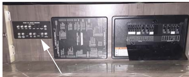
House Circuit Breakers -Typical View
