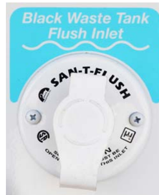
Black Waste Tank Flush Inlet (Located in water service center) -Typical View
