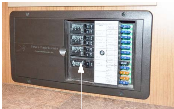
120-Volt Circuit Breakers -Typical View
