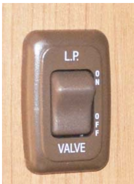
Main Tank Valve Switch (Located near monitor panel area) -Typical View
