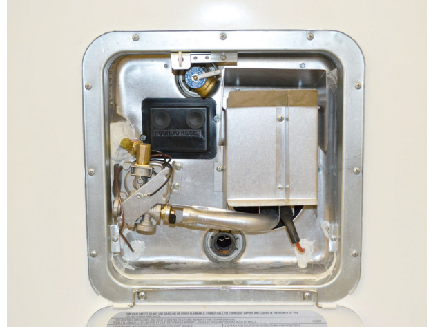
Water Heater Exterior Service Access
