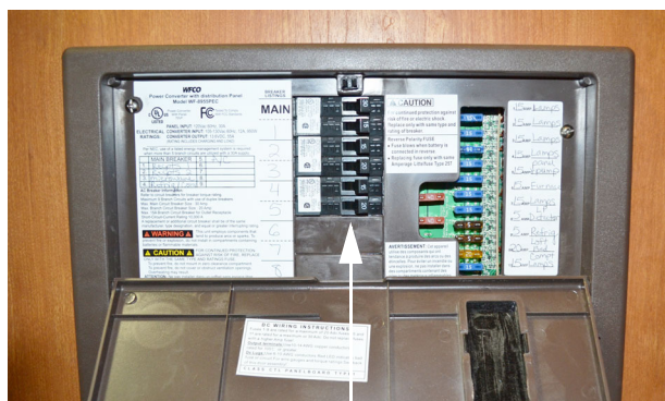
120-Volt Circuit Breakers -Typical View
