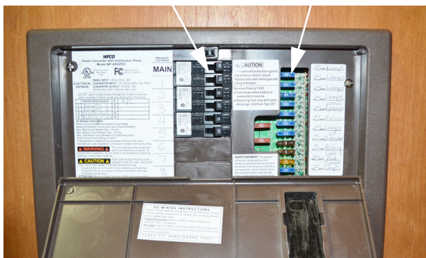
Power Center (Converter) -Typical View
