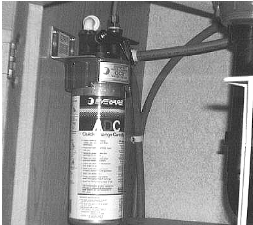
Water Filter Assembly - Below Galley Sink
