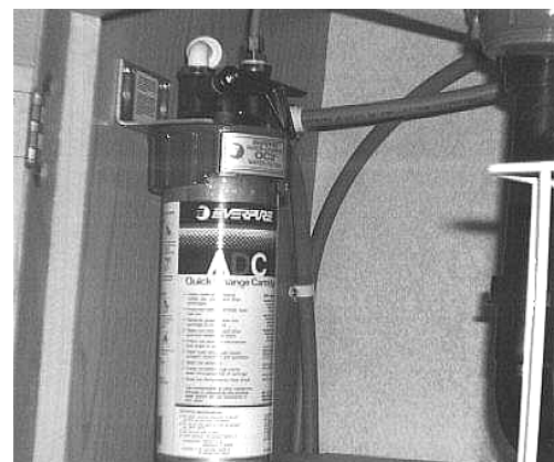
Water Filter Assembly - Below Galley Sink
