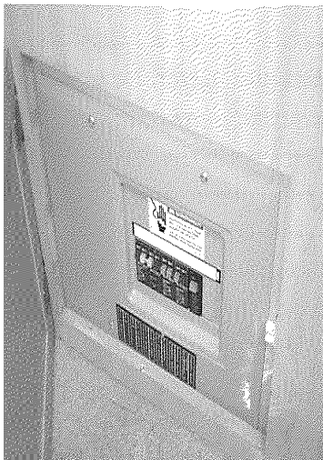
House 110-volt Breaker Panel
