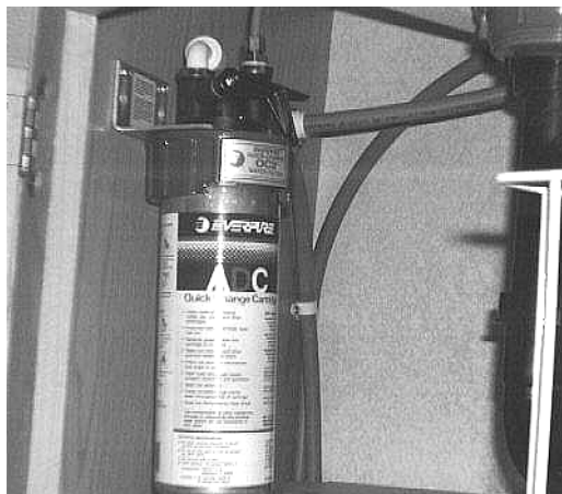
Water Filter Assembly - Below Galley Sink
