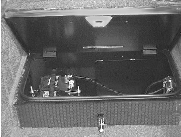
House Battery Storage in Entrance Step Models 27', 29' & 31'
