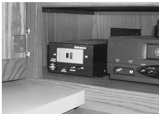
DC-AC Voltage Inverter in Video Center
