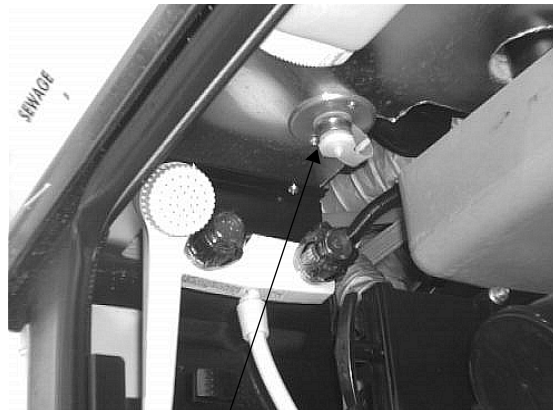
City Water Connection
