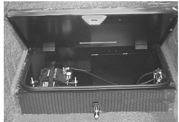
House Battery in Top Entrance Step
