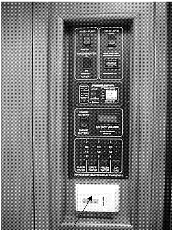
Power Vent Thermostat Bath Area
