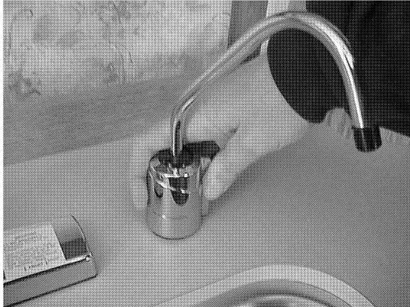
Water Filter Assembly - Below Galley Sink
