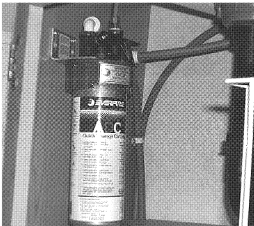
Water Filter Assembly - Below Galley Sink
