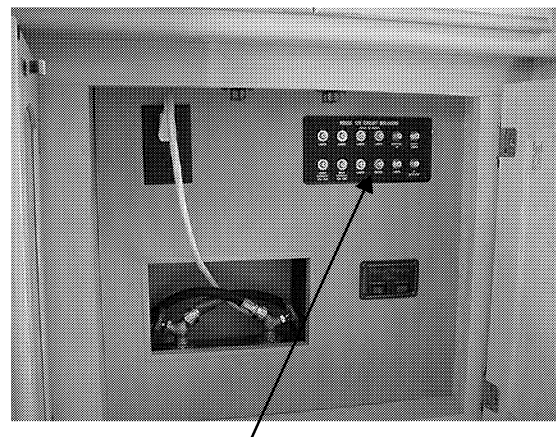
House 12V Breakers
