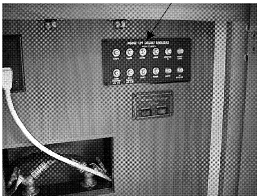
House 12-Volt Circuit Breaker Panel
