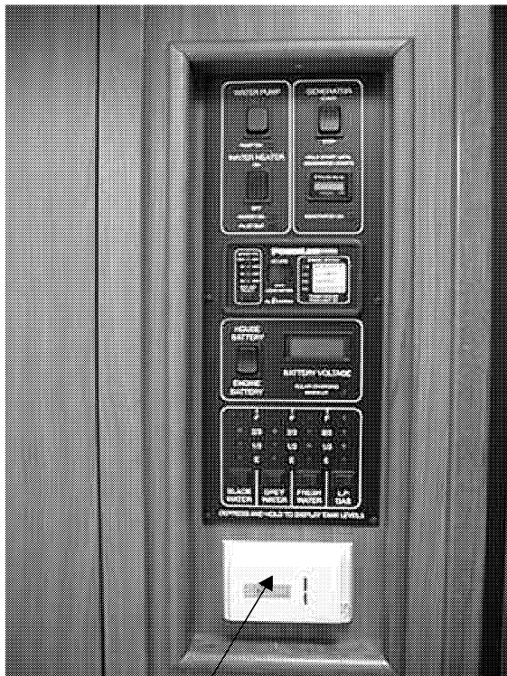
Power Vent Thermostat Bath Area
