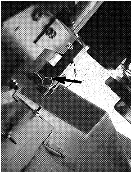
Travel Pin - see arrow Viewed looking downward at left side of generator through front “hood” panel opening.
