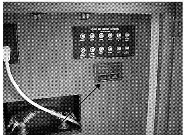
Winterization System Switches
