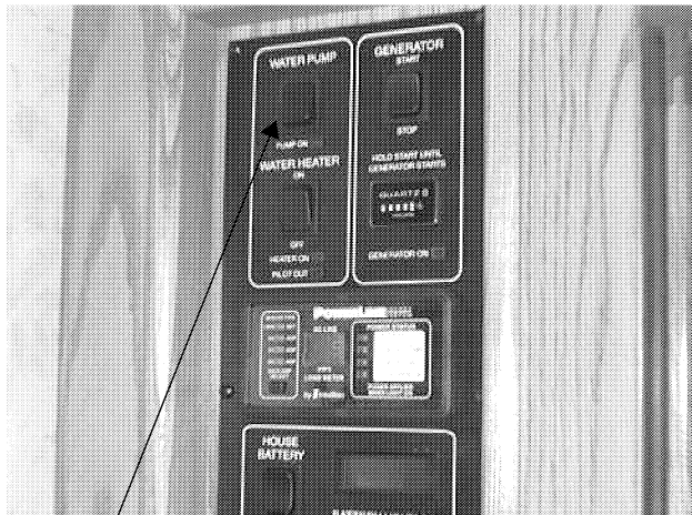
Water Pump Switch
