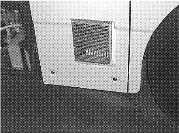
Water Heater Service Access Panel
