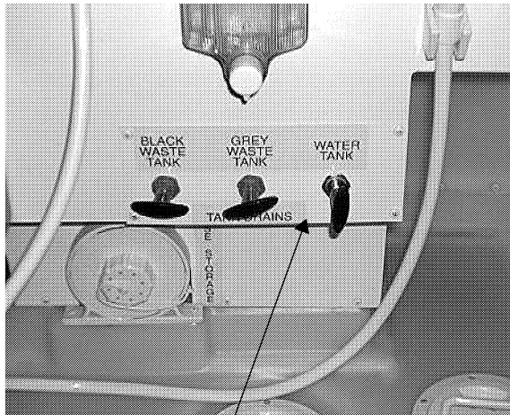
Water Tank Drain Valve (pull to open)
