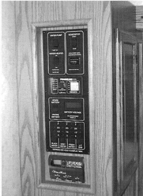
One Place Monitor Panel
