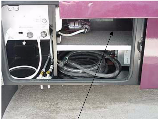
Inverter Charger Unit Location
