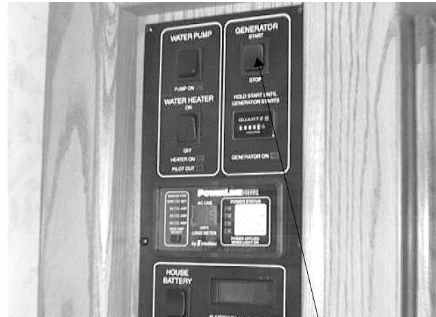
Generator Switch and Hourmeter
