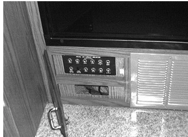
House 12V Breakers (below refrigerator)
