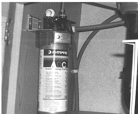
Water Filter Assembly - Below Galley Sink
