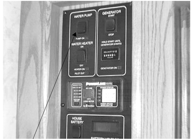
Water Pump Switch
