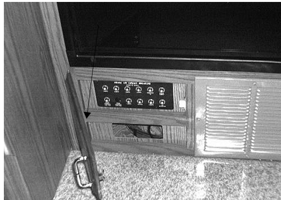
House 12-Volt Circuit Breaker Panel
