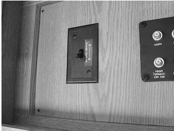
Electric Water Heater Switch (Typical)
