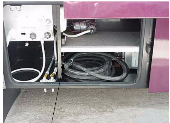
Water Heater By-Pass Valve
