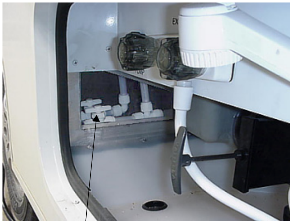
Hot and Cold Water Line Drains (in front of water service center)
