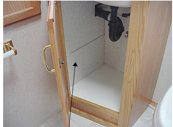
Water Heater Bypass Valve and Winterization Siphon Valve behind Access Panel beneath Bath Lavatory Vanity
