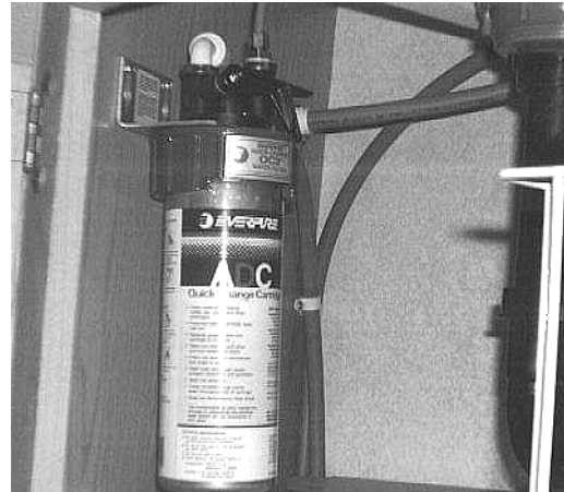
Water Filter Assembly - Below Galley Sink
