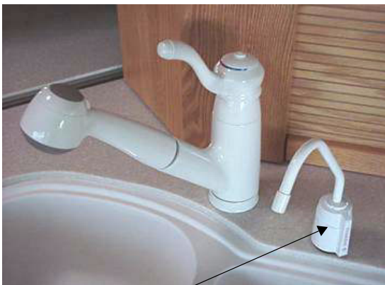
Filtered Water Faucet (Typical)
