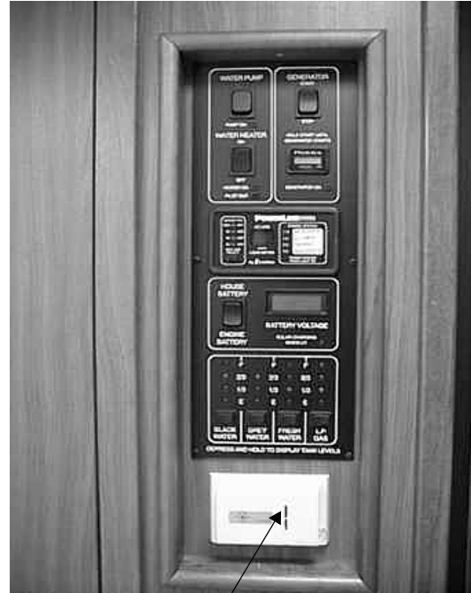
Power Vent Thermostat Bath Area
