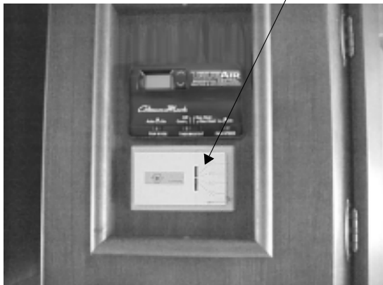
Power Ventilator Thermostat - Galley
