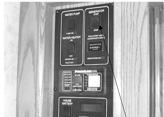
Generator Switch and Hourmeter
