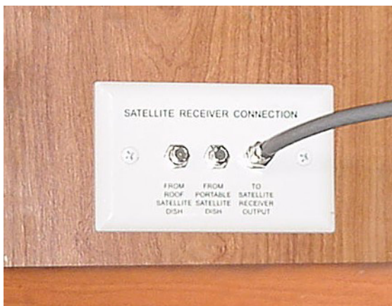
Interior Connection for Satellite Receiver
