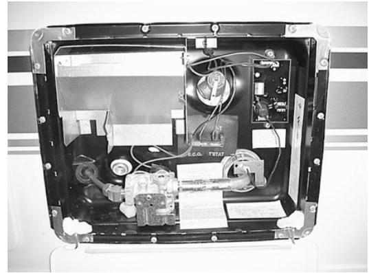
Water Heater Exterior Service Access
