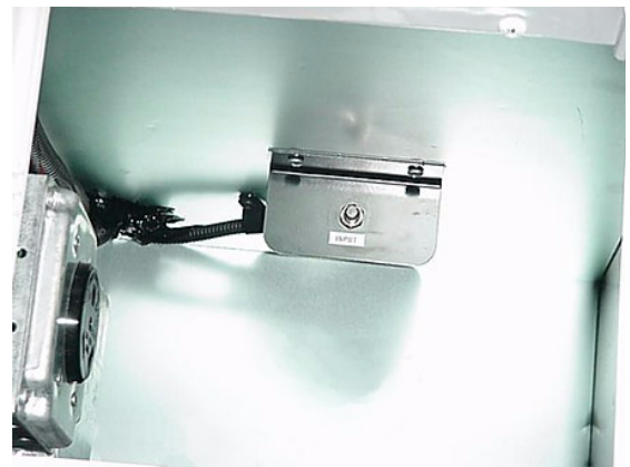
Cable TV Hook-Up in Utility Compartment
