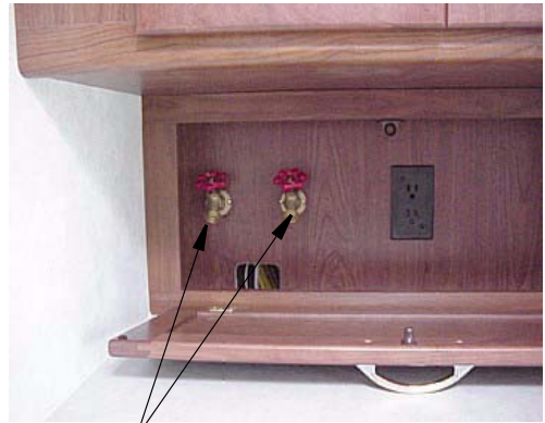
Water Supply Faucets -typical
