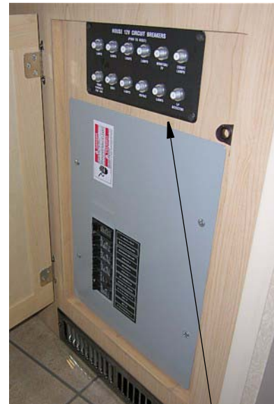
House 12-Volt Circuit Breaker Panel
