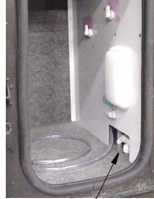
Water Line Drain Valve
