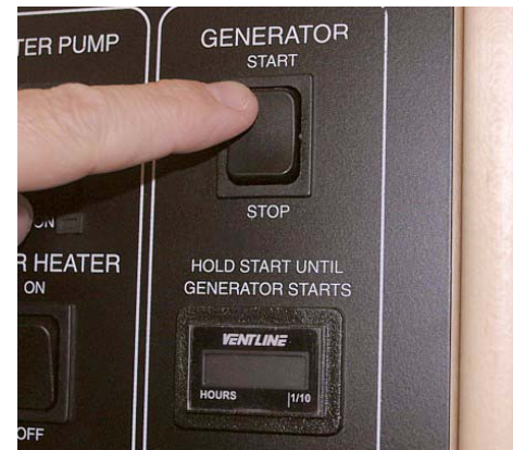
Generator Switch and Hourmeter on monitor panel
