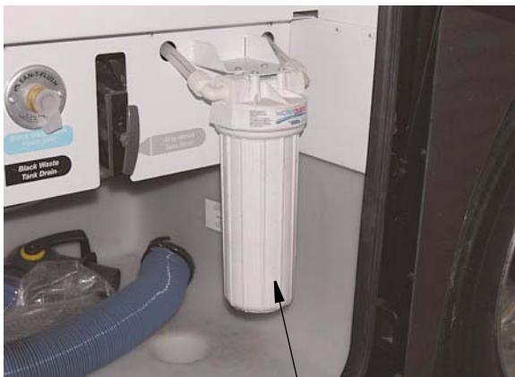
Central Water Filter System in Water Center (typical)
