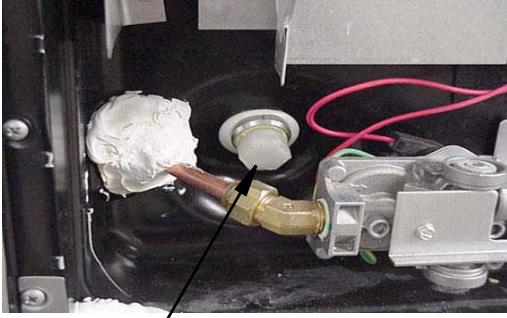
Water Heater Drain Plug (Remove with socket)
