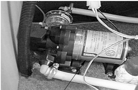
Water Pump (typical)
