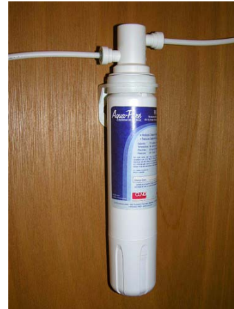
Water Filter Assembly below Galley Sink (Located below galley sink)
