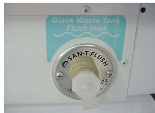
Water Tank Flush Inlet (typical)
