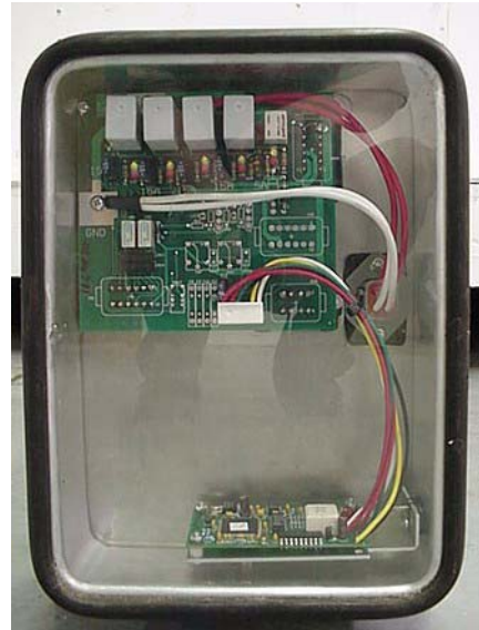
Hydraulic System Control Box on pump underside of coach near front tire
