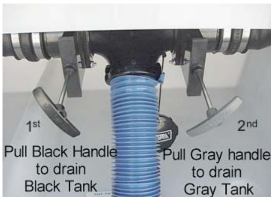
Holding Tank Dump Valves (Typical)
