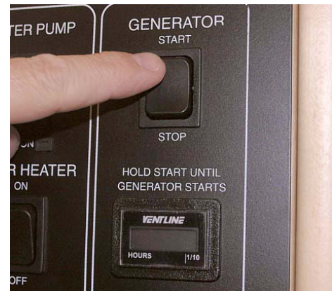
Generator Switch and Hourmeter on monitor panel
