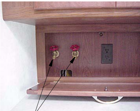
Water Supply Faucets -typical
