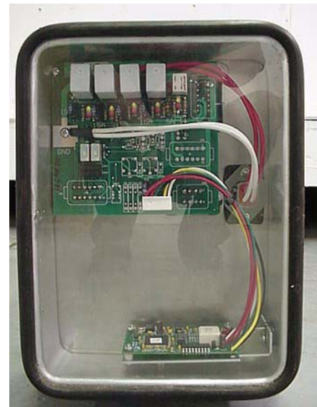
Hydraulic System Control Box on pump underside of coach near front tire
