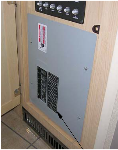
120-Volt House Circuit Breakers - typical
