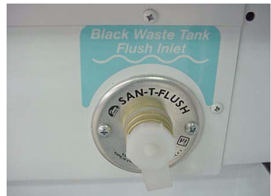
Water Tank Flush Inlet (typical)
