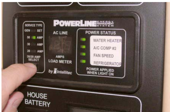
PowerLine EMS Display on Monitor Panel - typical
