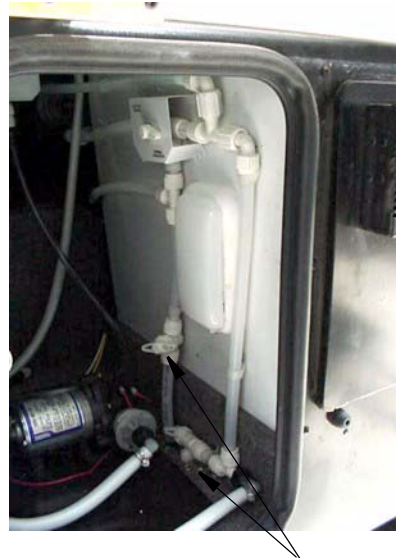
Water Line Drain Valves
