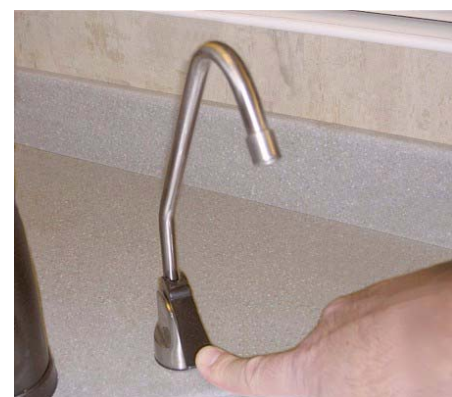
Filtered Water Faucet
