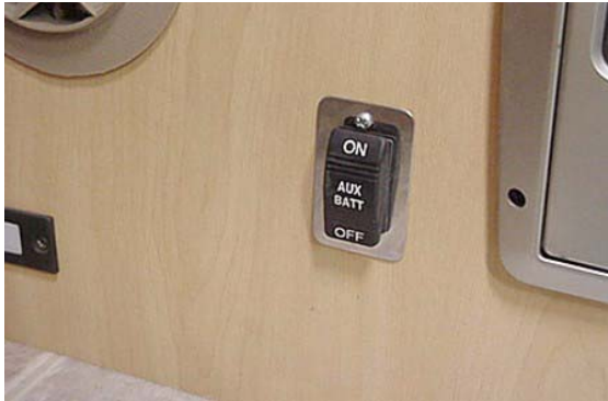
Aux. Batt. Switch - typical (Near entrance door)
