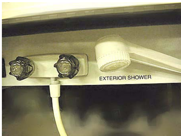
Exterior Shower/Wash Station (Typical)
