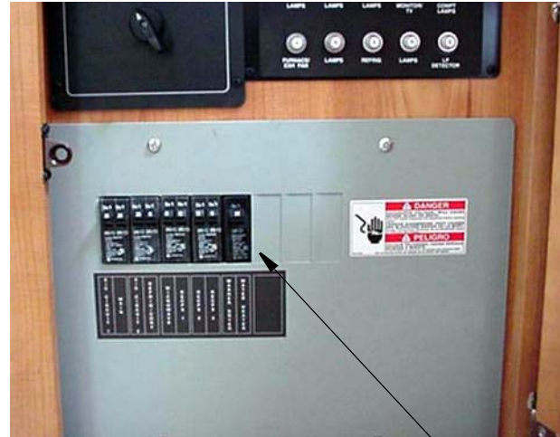
120-Volt House Circuit Breakers
