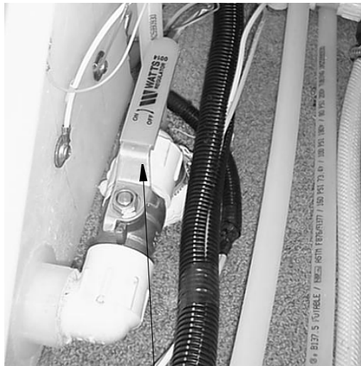
Water Tank Drain Valve (Typical)
