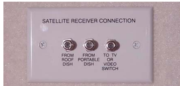
Satellite TV Receiver Connection (in front video center cabinet)
