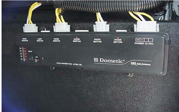
Awning Control Box (located in exterior compartment)
