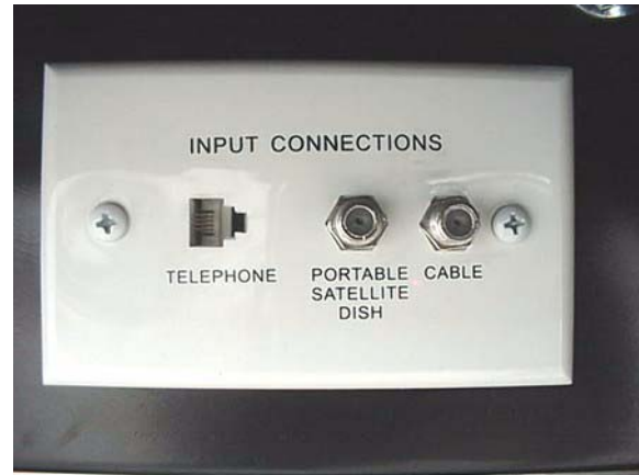
Exterior Connection for Satellite Dishes, Cable TV and Phone (in Water Center or Utility Compartment)
