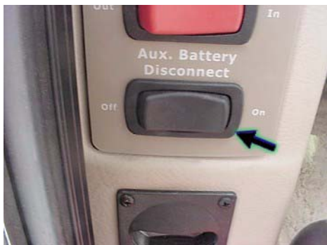
Aux. Battery Disconnect Switch (Near entrance door)
