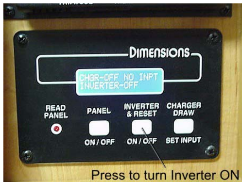
Inverter/Charger Control Panel
