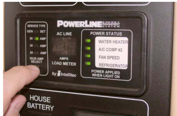
PowerLine EMS Display on Monitor Panel - Typical
