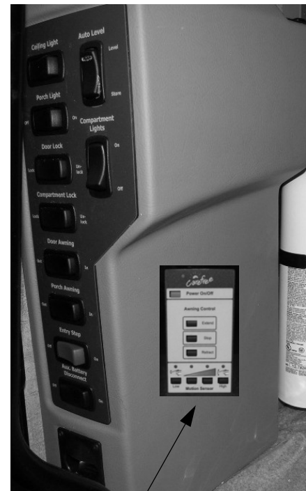
Awning Control Switch (Located just inside the entrance door)
