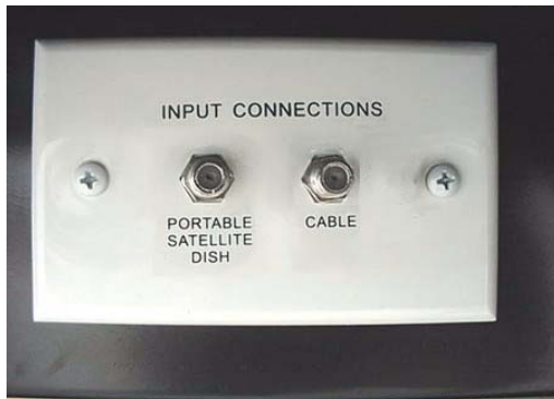
Exterior Connection for Satellite Dishes and Cable TV (In Utility Compartment)
