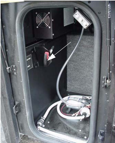
Water Tank Drain Valve - Model 38N shown (pull to drain) -Typical View
