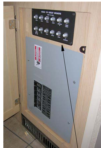
House 12-Volt Circuit Breaker Panel
