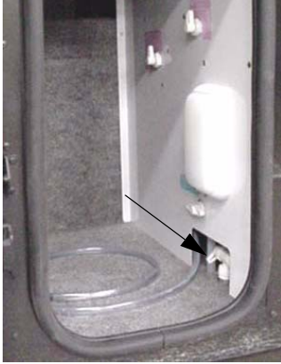
Waterline Drain Valve -Typical View
