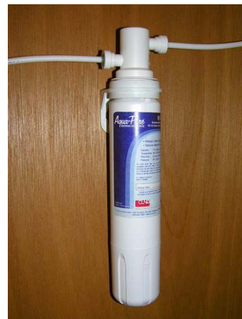
Water Filter Assembly below Galley Sink
