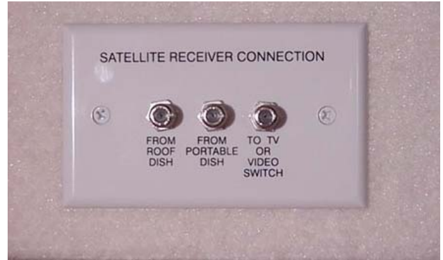
Interior Connection for Satellite Dishes (Located in cabinet near TV) - Typical View
