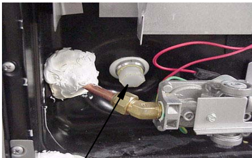
Water Heater Drain Plug Remove with socket
